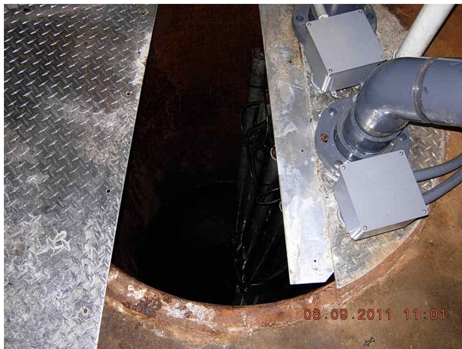
Figure 55. Views of the second VA Hospital sanitary lift station, also located inside one of the buildings. A noticeable sewage odor with ammonia prevailed. The pump station is sealed.
