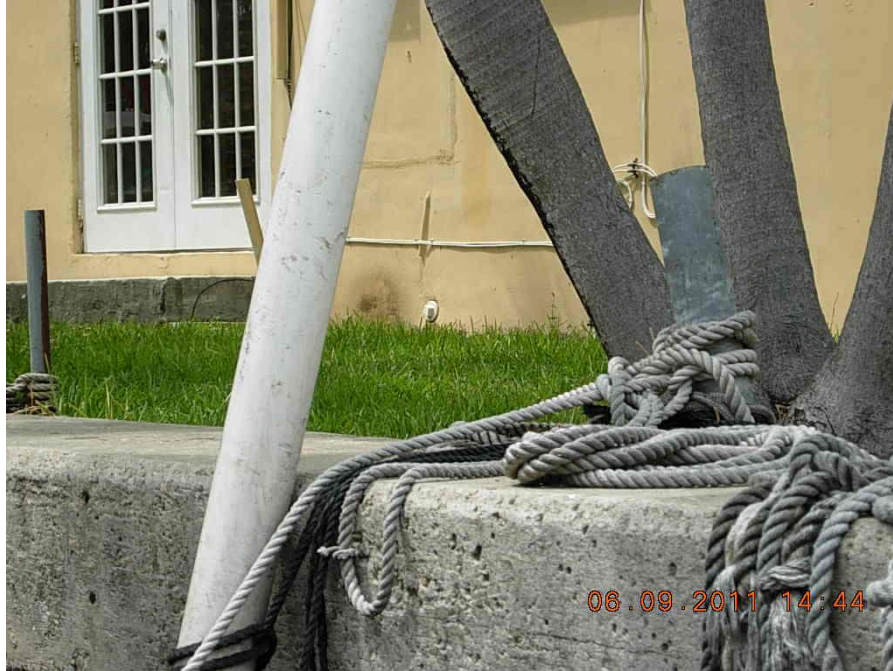
Figure 79. A capped lateral (possibly sanitary) at what appeared to be an apartment house. The approximate address is 938-942 NW 8 th Street. GPS coordinates are 25 46' 57.495" N, 80 12' 31.280" W.
