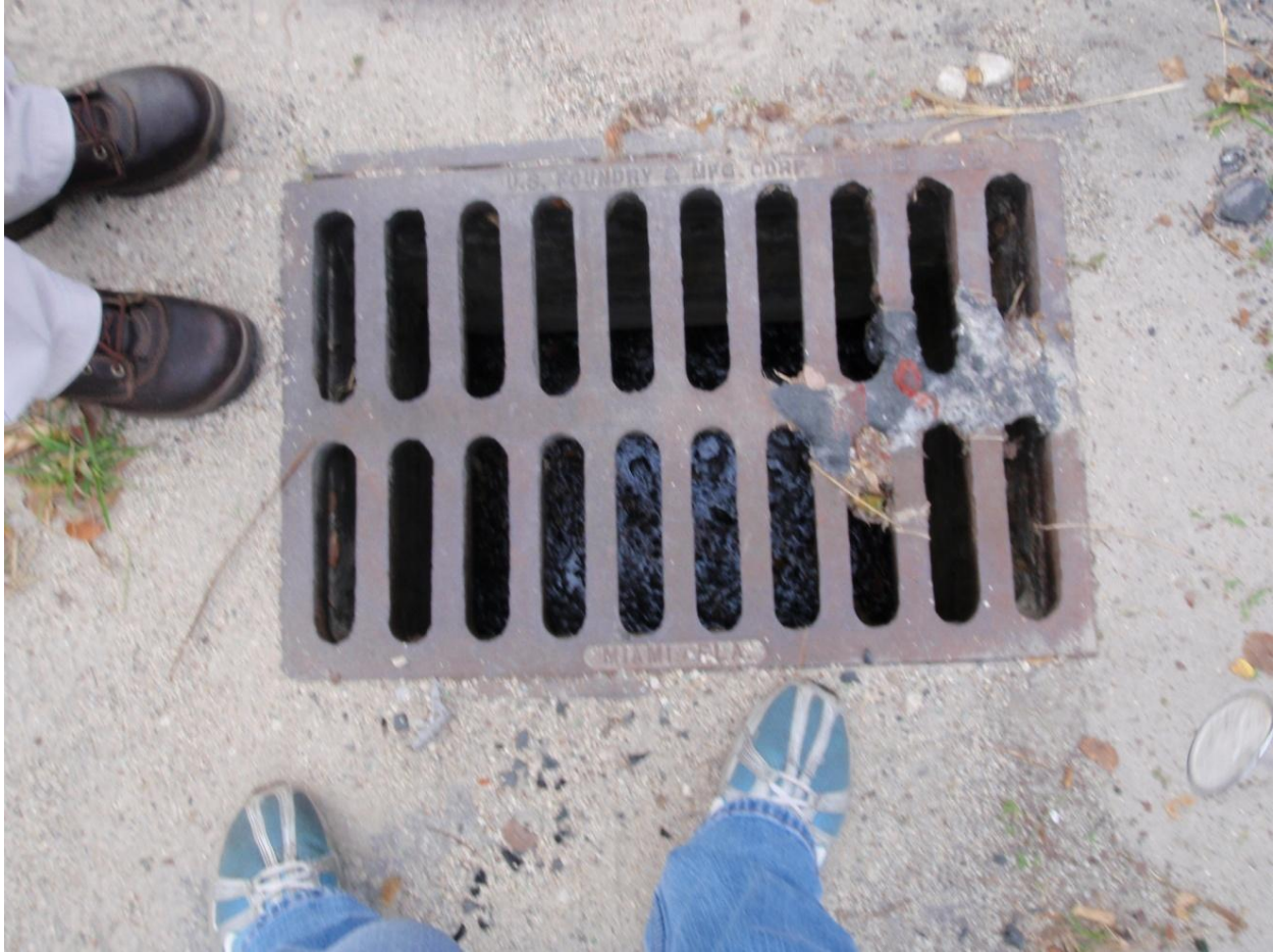
Figure 20. A storm drain on NW 15 th Avenue south of NW 20 th Street is filled with trash and not draining properly; any flooding that results could cause a failure of the wastewater system, and trash can provide a breeding ground for fecal coliform.
