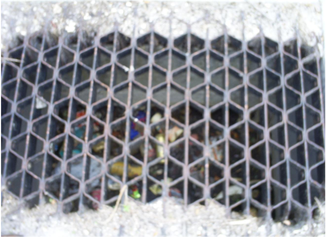
Figure 42. Litter, debris, and trash in a stormwater drain inside the Miami–Dade Transit Culmer Metrorail Station in the Highland Park area.
