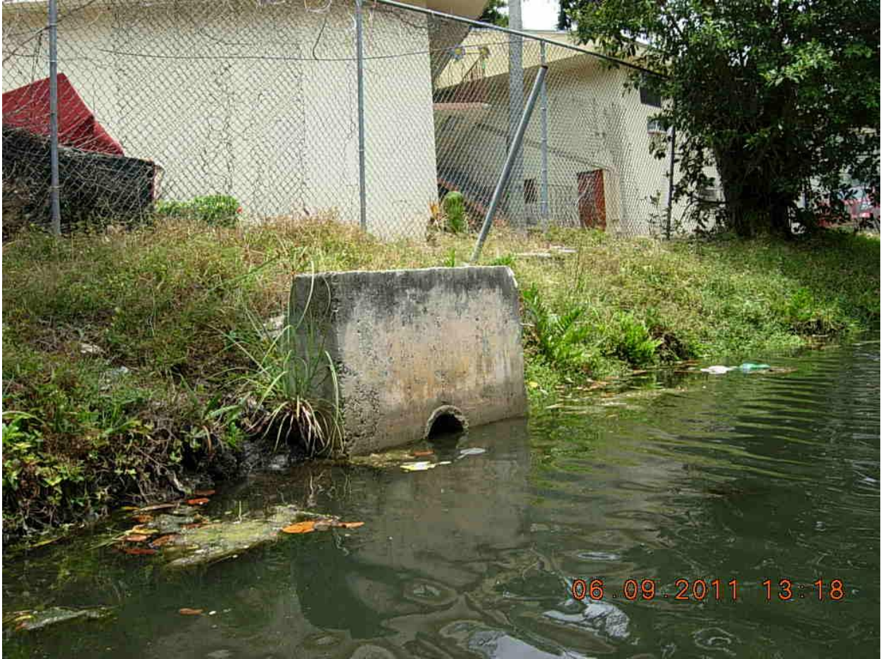
Figure 63. The first PIC was an 8-inch-diameter concrete pipe with a headwall. GPS coordinates are 25 47' 37.142" N, 80 13' 15.892" W.
