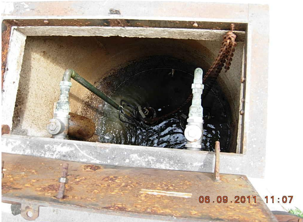
Figure 56. Views of the VA Hospital sanitary lift station located outside between Buildings 8 and 9. The pump station appeared relatively clean. No grease was observed.
