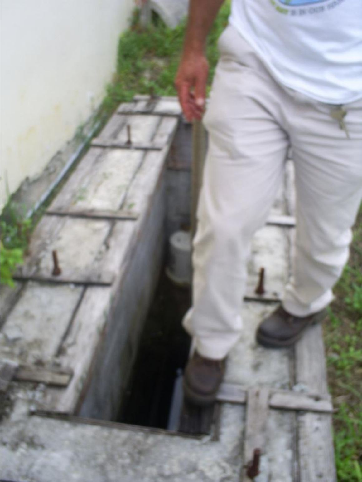
Figure 46. A PIC at the City of Miami Overtown stormwater pump station consists of those portions of the incomplete upgrades that allow foreign objects to enter the stormwater system.
