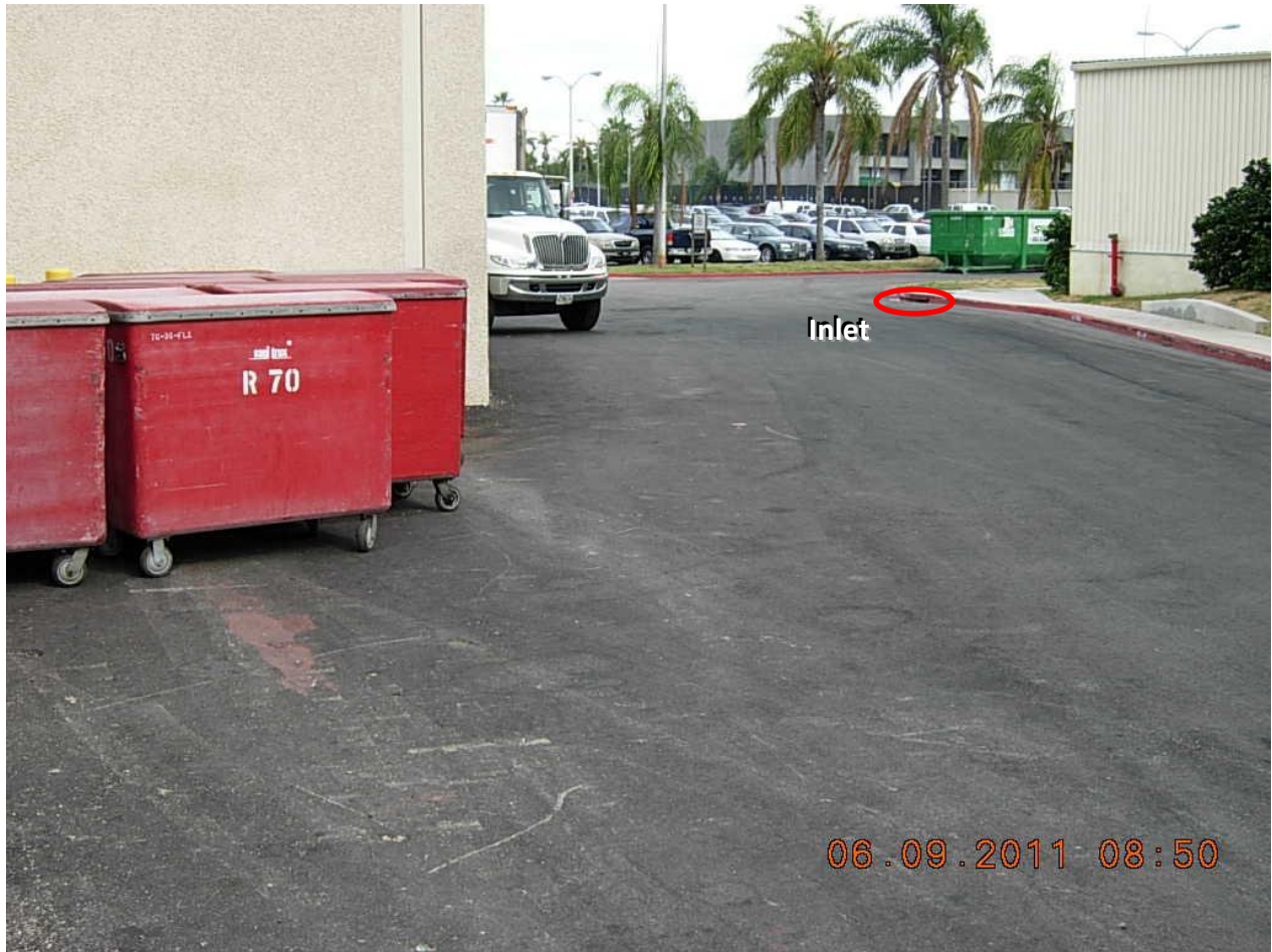
Figure 53. View of a portion of the VA Hospital site, near the western parking lot. On the way in to inspect the sanitary lift stations, the team observed closed biomedical waste bins upstream of the curb opening inlet (circled in red at top right). One of the team members observed some small holes in the bins. In the same area, a roll-off container was observed upslope of a drop inlet (at left).
