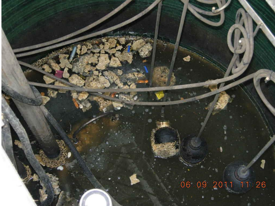
Figure 59. Interior of the new lift station.
