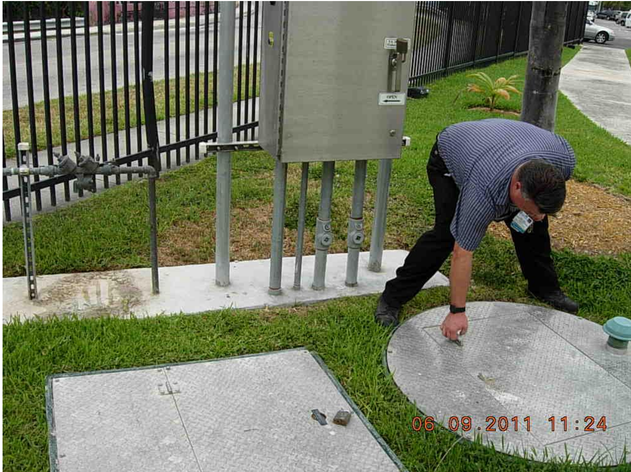
Figure 58. View of the fourth VA Hospital sanitary lift station near NW 17 th Street, close to the newly completed Fisher House. The Wagner Creek guardrail is just visible in the upper left corner of the photo. This is a new lift station that had not yet completed the DERM permitting process at the time of inspection. Scott Olsen of the VA Hospital opened the pump station. Debris and some globules were observed. Allen Cox from DERM suggested pumping out the new station.
