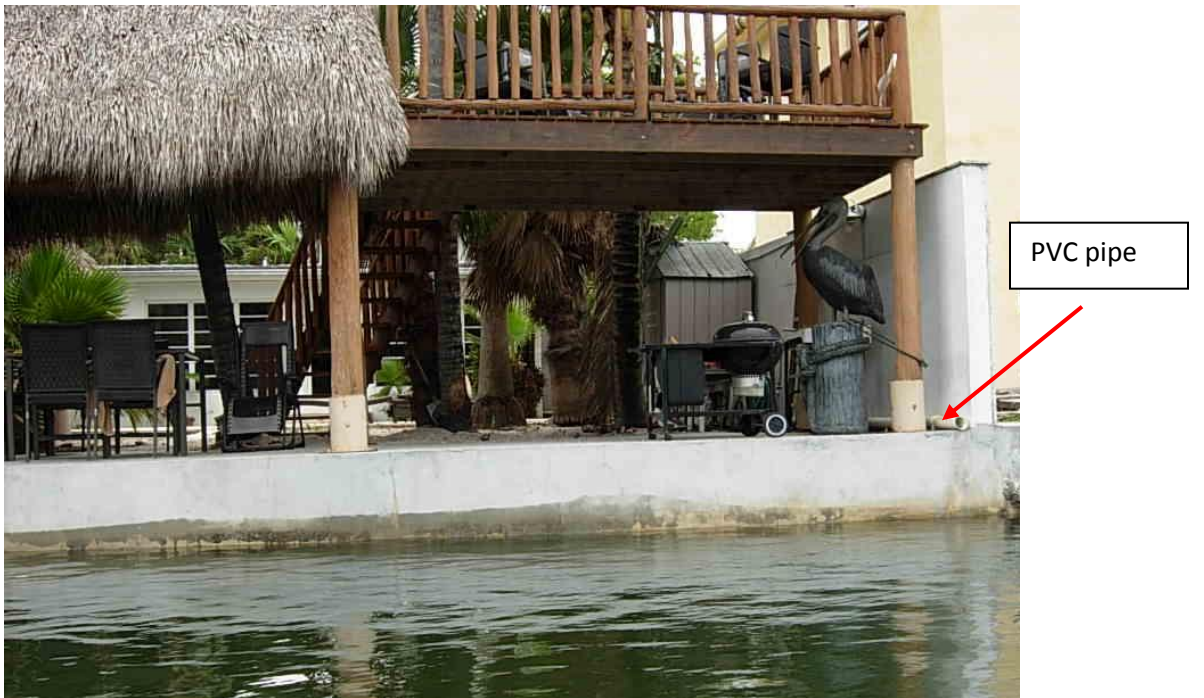
Figure 81. At 727 NW 7 th Street, the team observed a 4-inch white PVC pipe running from the property line at Seybold Canal towards the front of the property.
