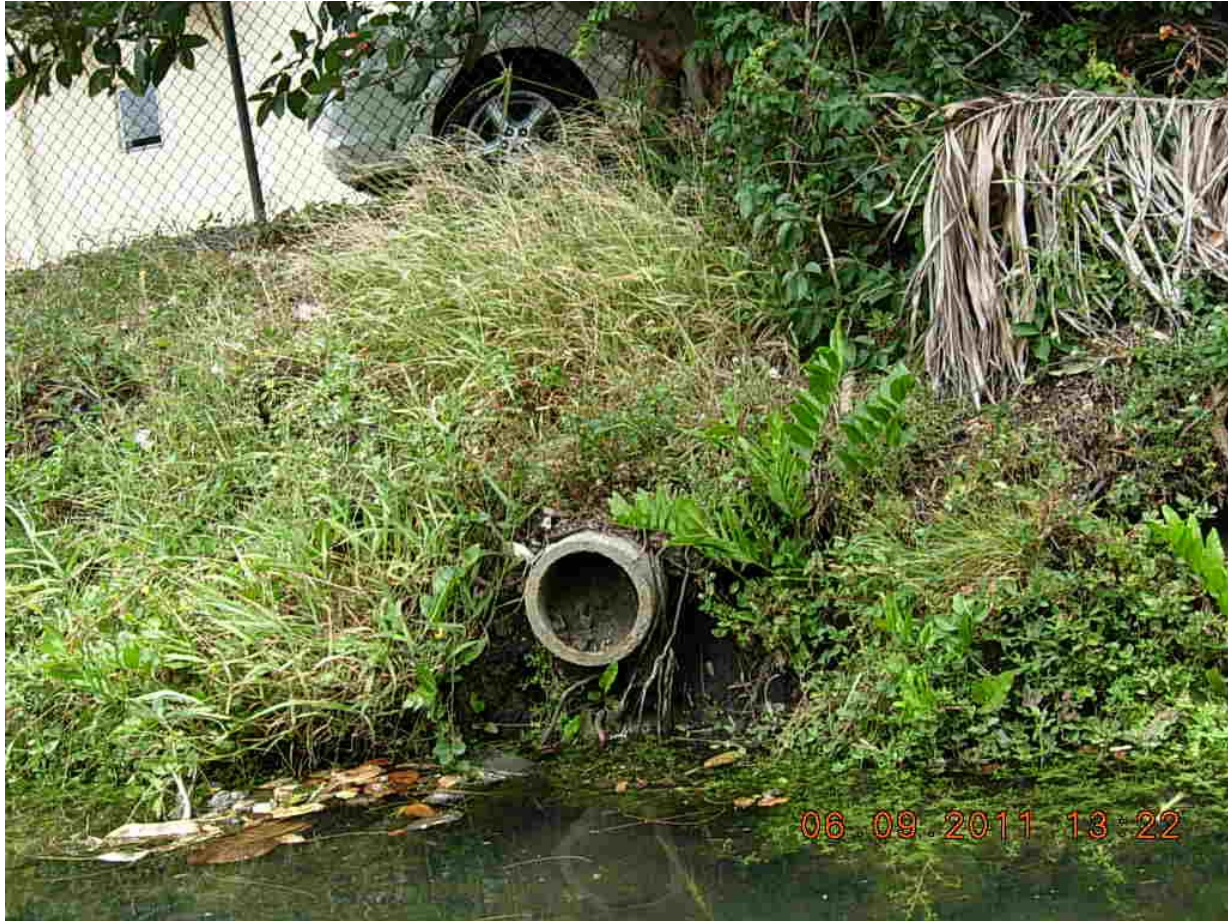
Figure 65. Another 8-inch diameter concrete pipe, without a headwall, was located farther to the south and appeared to belong to the same apartment complex. The outfall was full of sediment. GPS coordinates are 25 47' 36.299" N, 80 13' 14.842" W.
