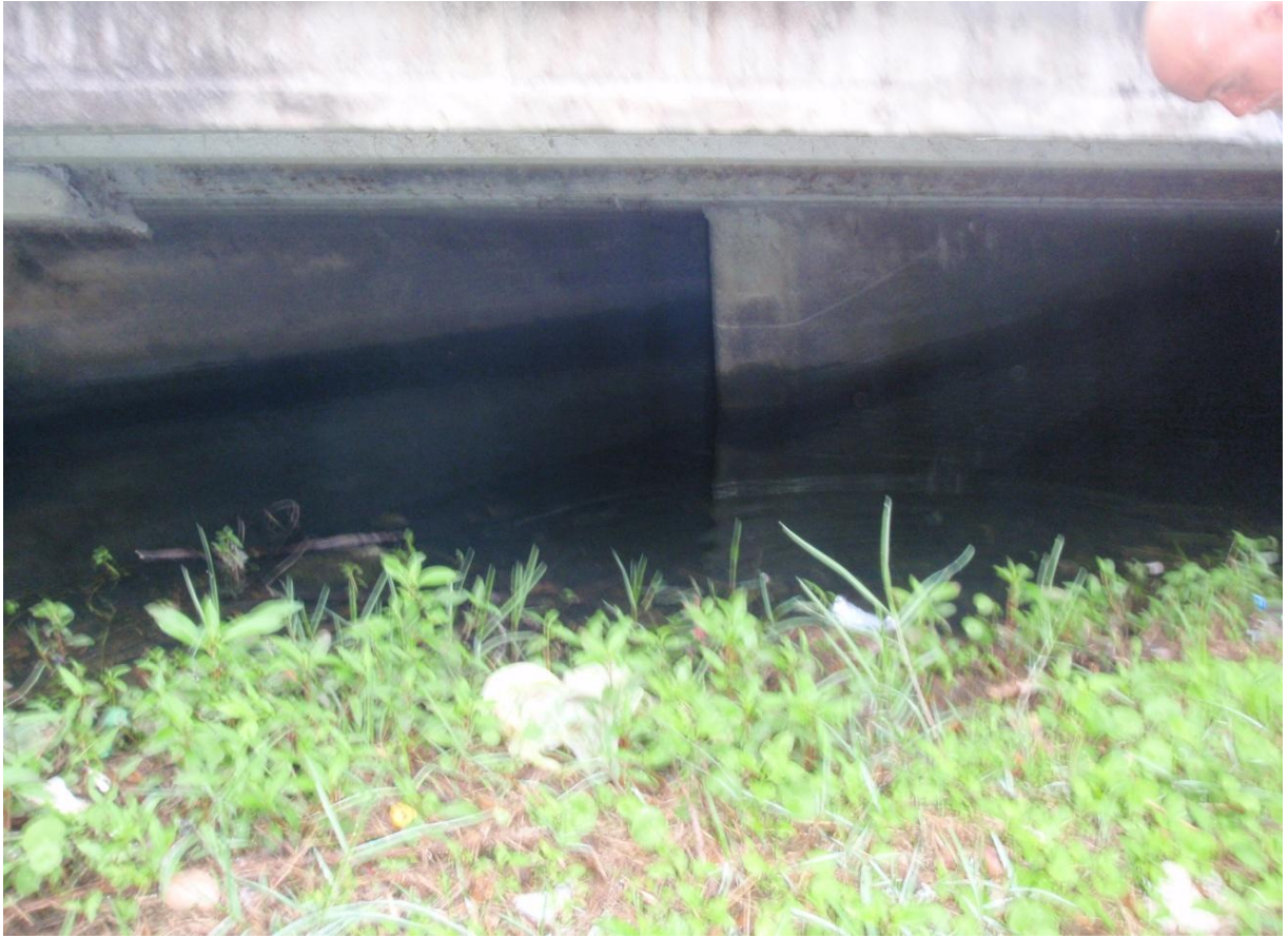
Figure 5. View of stagnant water and trash buildup in the stormwater conveyance that flows underground to the 20 th Street Bridge; the accumulation may be caused by a blockage and should be investigated. This may be where the perennial portion of Wagner Creek now begins.
