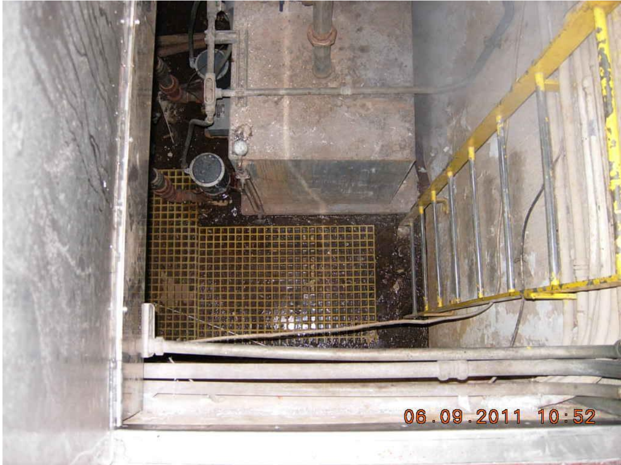
Figure 54. View of the first VA Hospital sanitary lift station, located inside one of the buildings. The VA staff stated that the pump station was “open” rather than “sealed” because it is located in an area where there is a continuous flow of air from outside. Harold Moesch from FDEP entered the pump station for a closer investigation. No unusual conditions were observed. There was a noticeable mercaptan odor at this location.
