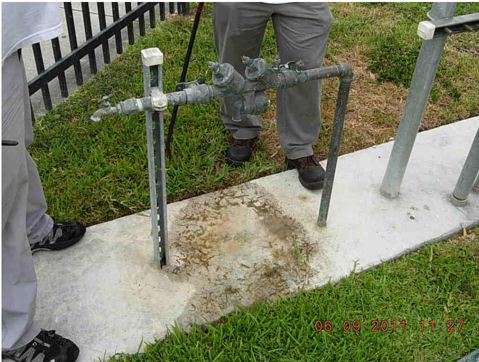
Figure 60. Close-up view of slowly leaking backflow preventer at the lift station.
