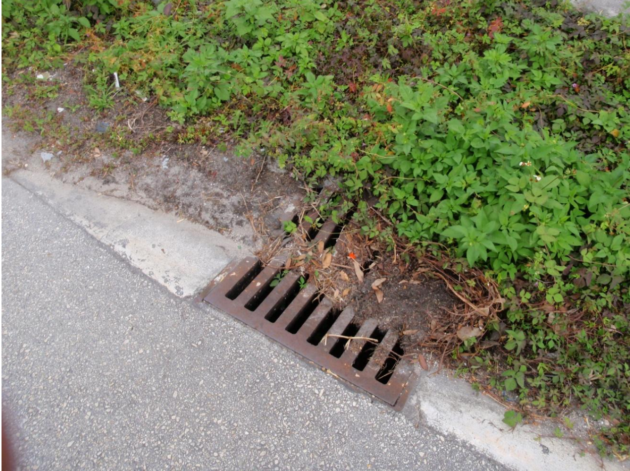
Figure 25. View of a partially blocked stormwater drain at 1501 to 1511 NW 13 th Court; any flooding that results could lead to the failure of septic and wastewater infrastructure.
