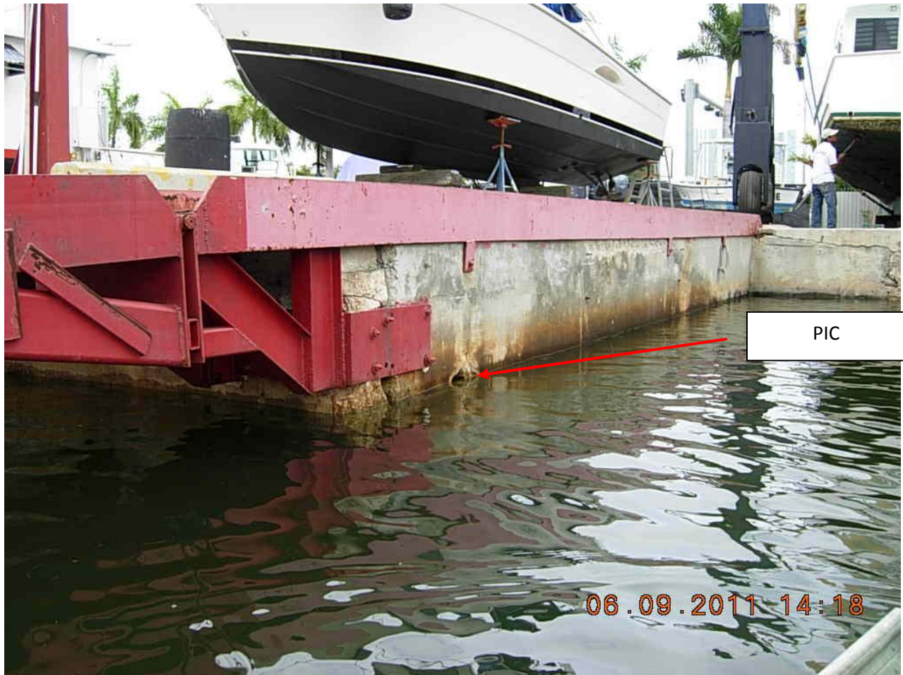
Figure 71. PIC observed at Campeones Boatyard, 600 NW 7 th Avenue. GPS coordinates are 25 46' 45.720" N, 80 12' 25.987" W.
