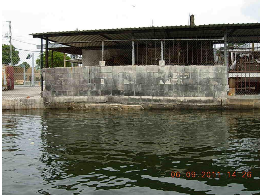
Figure 75. At 732 NW 7 th Avenue, the team observed a concrete structure that may be a submerged outfall. The structure could not be observed in its entirety. GPS coordinates are 25 46' 50.661" N, 80 12' 26.025" W.
