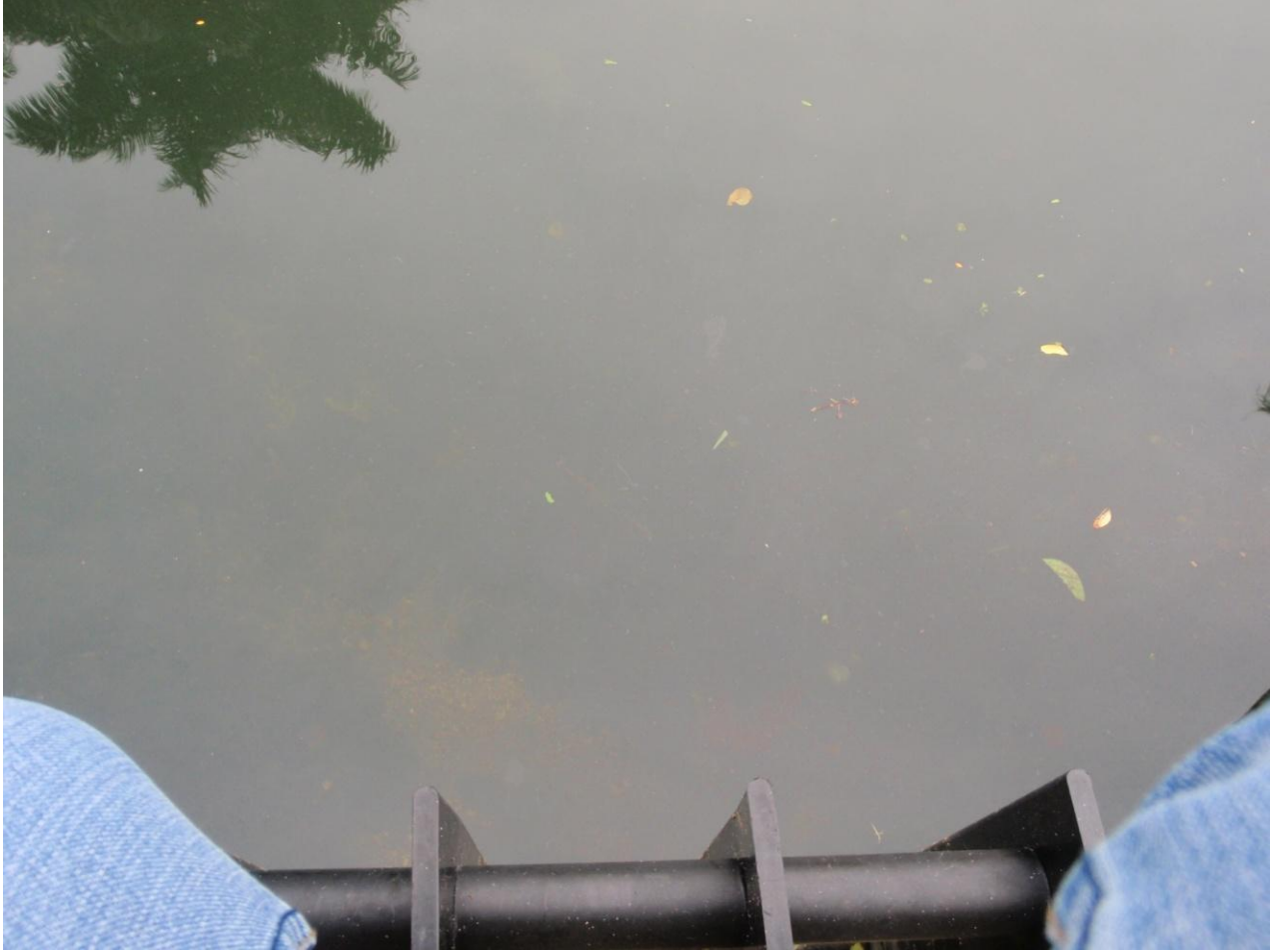
Figure 32. Solids and oils floating on surface water at a stormwater outfall from the VA Hospital building.
