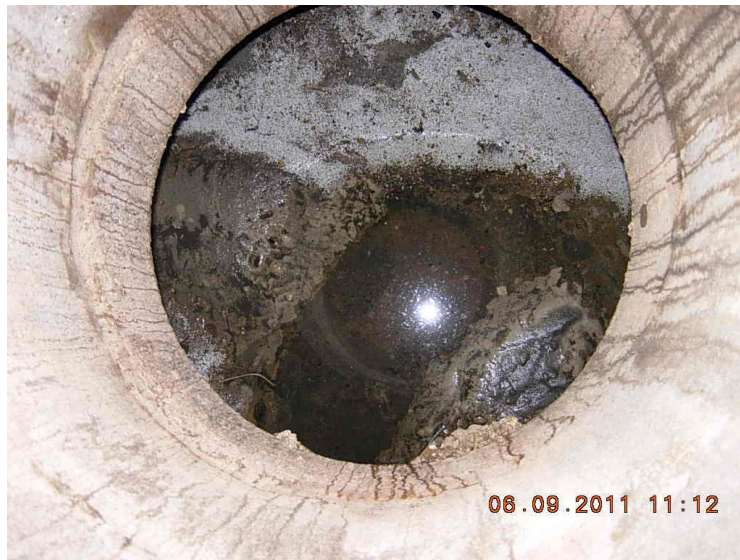
Figure 57. Views of the storm sewer manhole located around the corner from the VA Hospital's third pump station near the Endocrine, Polypeptide, and Cancer Institute. Upon inspection, no sanitary sewage impact was observed at this manhole.
