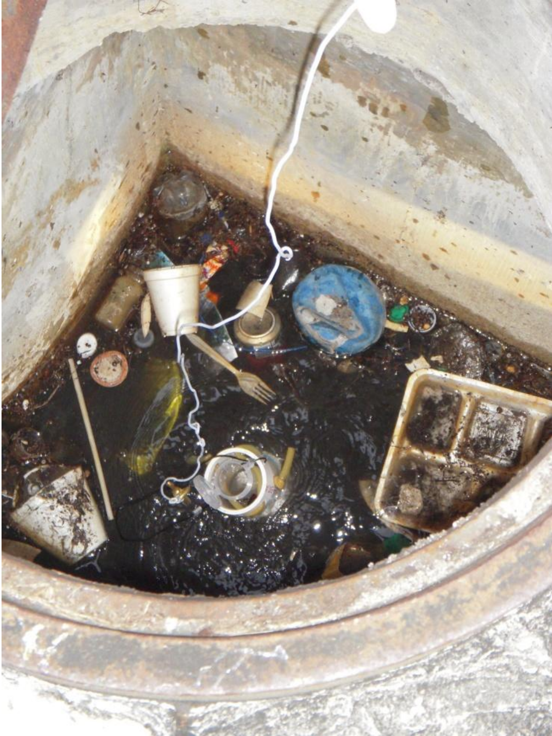
Figure 3. Trash and debris in a stormwater manhole thought to be at the headwaters.
