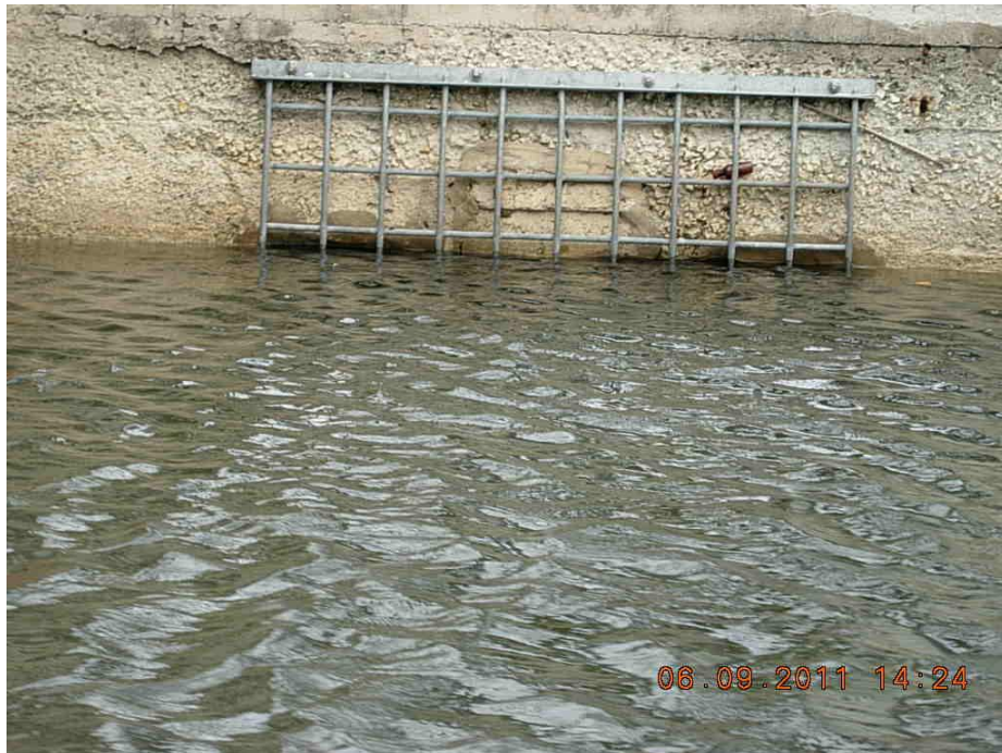
Figure 74. A sealed outfall with a manatee grate at NW 7 th Avenue and NW 7 th Street. No GPS coordinates were taken.
