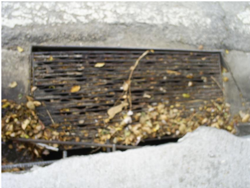
Figure 19. Broken storm drain covers at NW 20 th Street belonging to Miami–Dade County; the openings allow trash and other materials to enter the underground conveyance directly and provide a breeding ground for fecal coliform.
