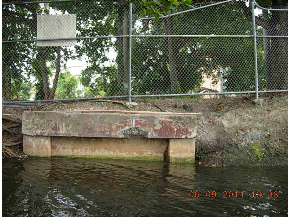
Figure 68. A submerged outfall that appears to be from the public storm sewer system is located across the street from NW 19 th Terrace near the put-in point.
